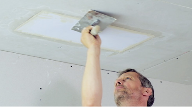
Plaster twice over the edges and drill holes. Leave to dry for at least 24 hours!
