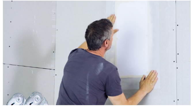
Attach the lining while the adhesive is still moist. Press with your hand or a dry roller. Leave to dry for at least 24 hours!
