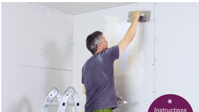
Apply 1-2 thin layers of plaster over the entire surface. Leave to dry for at least 24 hours!
