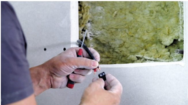
Attach the terminal to the speaker cable. Make sure the polarity is correct.
