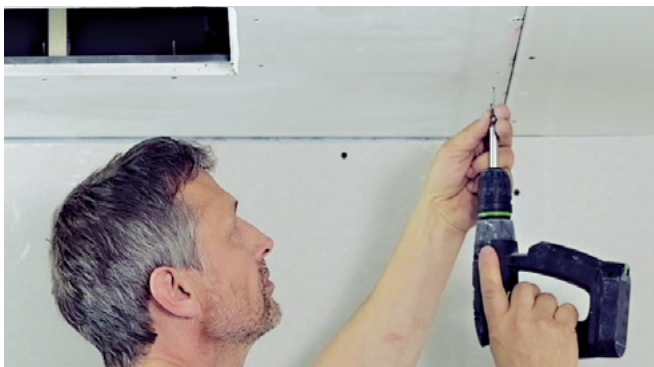
and screw the drywall sheet into the ceiling. Seal the cable hole in the back box.
